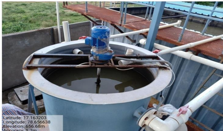
Mixer Pump and Tank, Removal of Floating Settlable Materials
