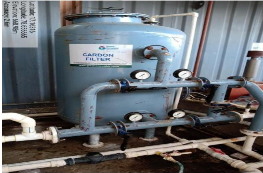
Carbon Filter Removes Chlorine from Water Waste
